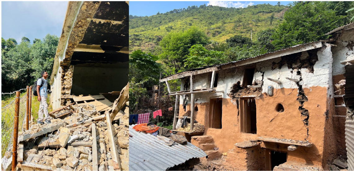
A damaged school building (left) and an example of a damaged house (right) from the Bajhang Earthquake.
